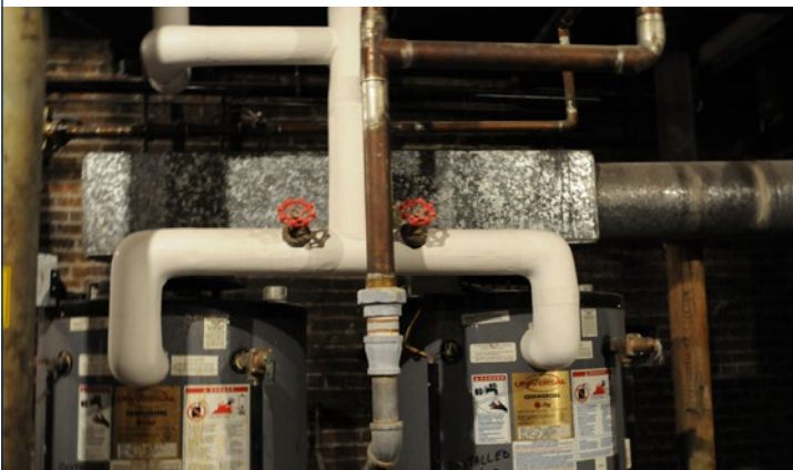
Figures 6 and 7: Elevate Energy recommended insulation for the heating pipes in the basement.
