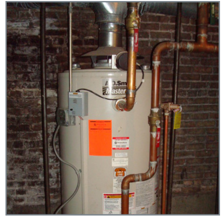
Water heater at 2212-2214 N. Sacramento Ave./3001 - 3003 W. Lyndale St.
