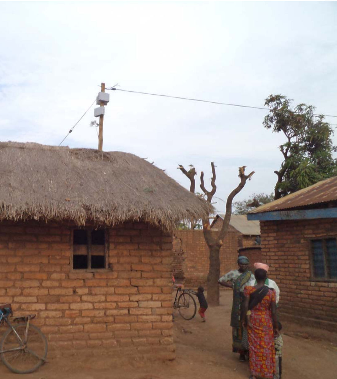
Pole-mounted metering boxes on an off-grid microgrid in Tanzania.
