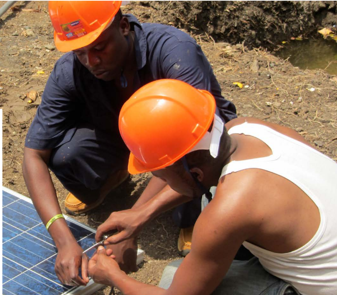
Peter and Talbot getting a panel ready for installation on the Organic Health Response Clinic roof on Mfangano Island.
