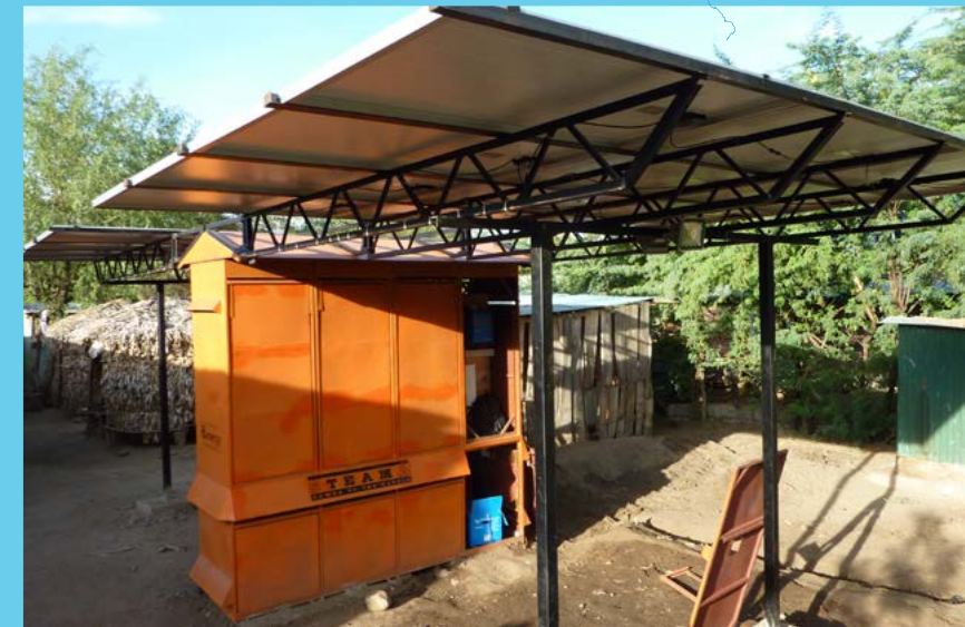
The Power Hub at Entesopia contains all the energy storage and control technology.
