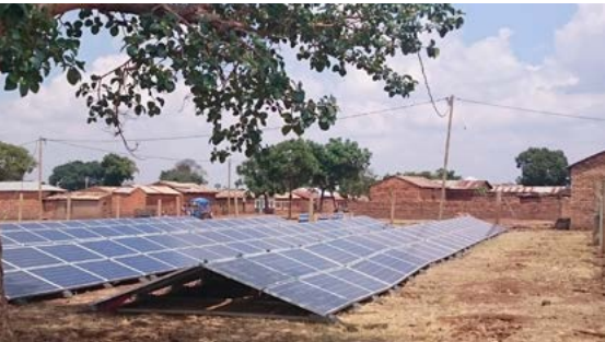
A sizeable PV array provides power for a large village in southern Tanzania.
