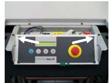
Control panel closed
