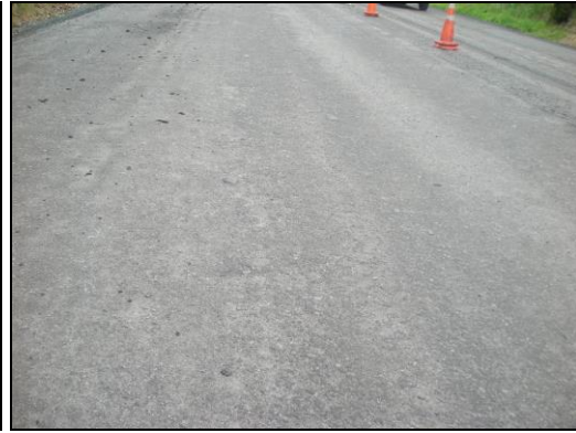
Exposed FBS basecourse prior to reseat
