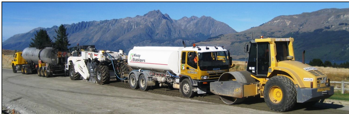
FBS 'train' operating in Queenstown illustrating from left to right bitumen tanker, WR2000 purpose-built hoe, water tanker and primary steel drum compaction plant.
