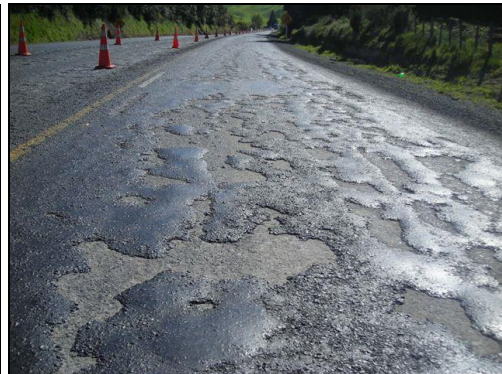
October '07 major surfacing failure
