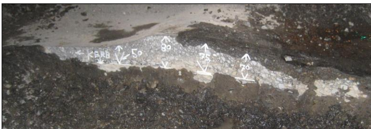
Trenching by the Client confirmed relief was entirely in membrane / asphalt surfacing with a level FBR surface
