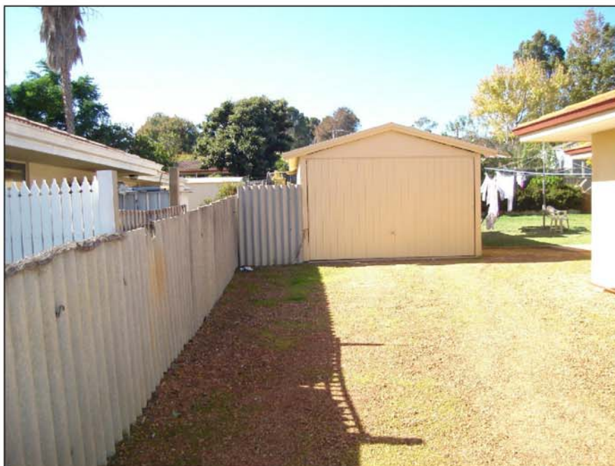
PHOTOGRAPH 2 EXISTING ASBESTOS SHED TO BE REMOVED ON LOT 105 SCHRUTH STREET NORTH, KELMSCOTT
