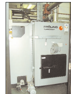
The Froling boiler
