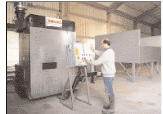
The Talbott's B3 boiler and feed hopper
