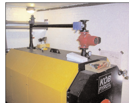
220 kW wood pellet boiler
