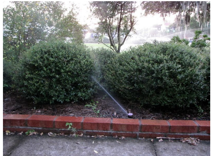
Figure 3. Blocked water spray (photo by Bernard Cardenas).
