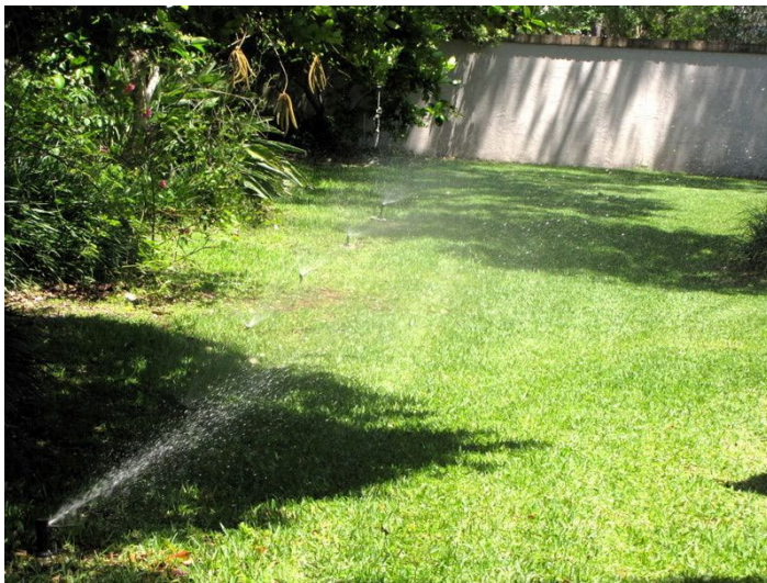
Figure 2. Mixed sprinkler types. Note: rotary sprinkler in foreground and spray heads in background (photo by Bernard Cardenas).
