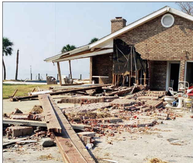
Figure 2-11. Example of surge, wave, and debris damage. (Source: FEMA 489)
