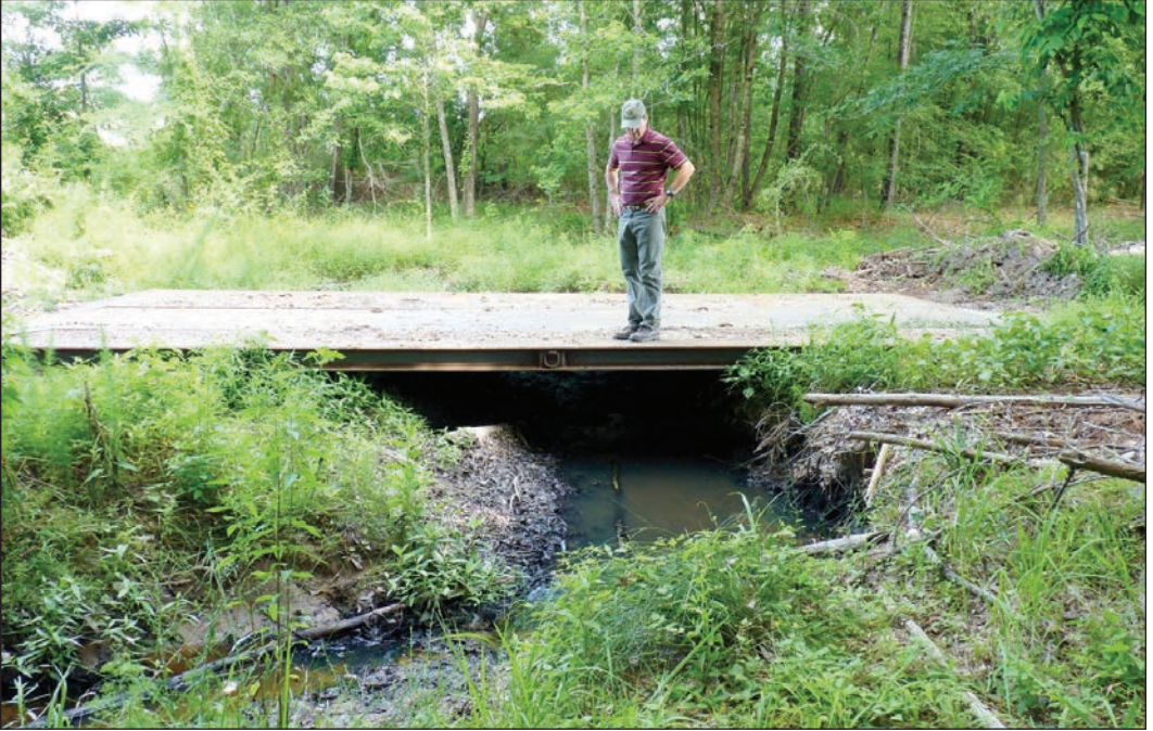
Installation of temporary bridges like this metal one can be used on temporary forest roads.
