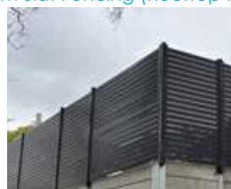
Alum Slat Fencing (Rooftop Plant)
