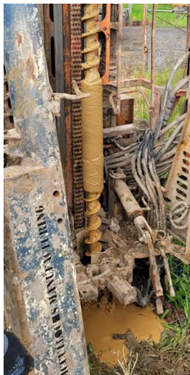
Photo 8 - Water encountered at BH14 (23/05/2022)
