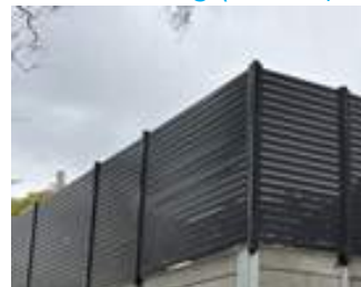
Alum Slat Fencing (Rooftop Plant)
