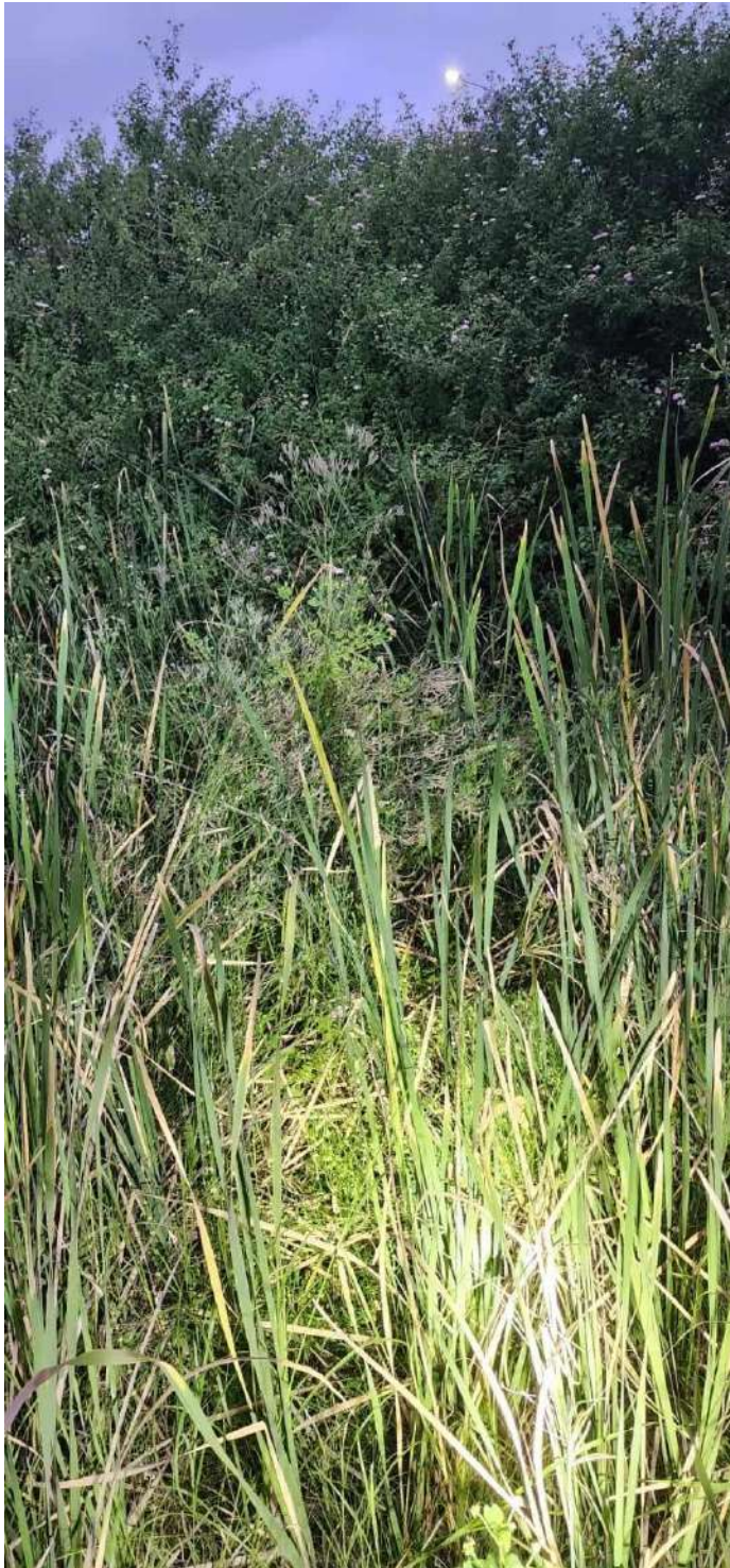
Figure 3. This is the location of two culverts. They are completely obscured by vegetation and are unsuitable flight paths for Microbats.
