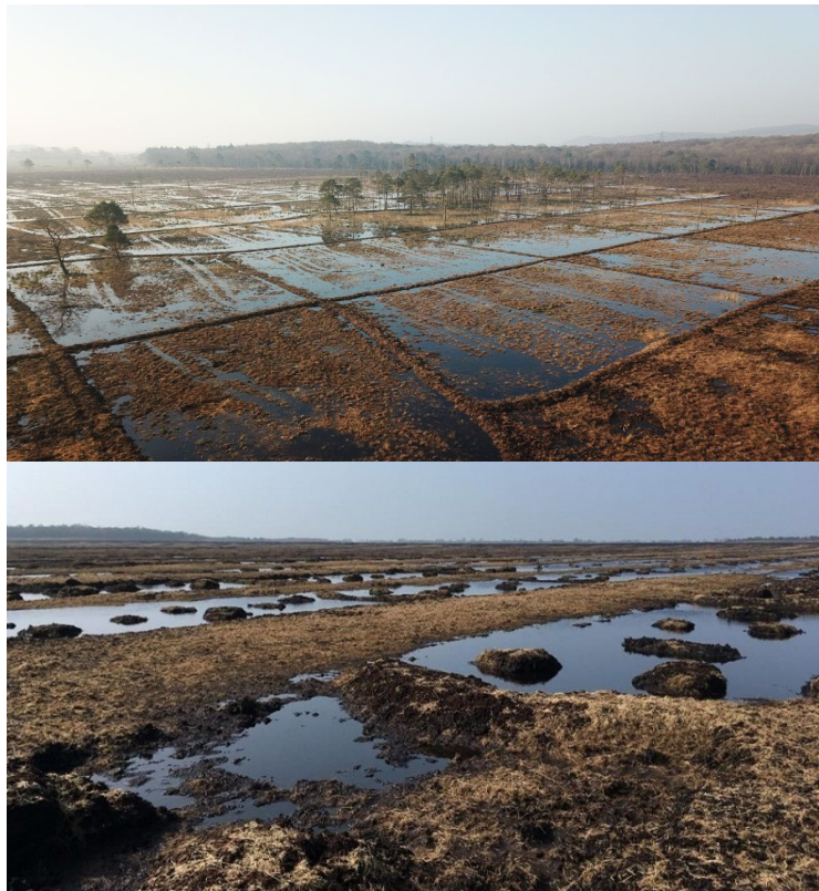
Figure 9 Top: Cell bunding at Roundsea woods & Mosses NNR. Photo Credit: Conservfor. Bottom: Horseshoe bunds at Bolton Fell Moss. Photo Credit: Deborah Land
