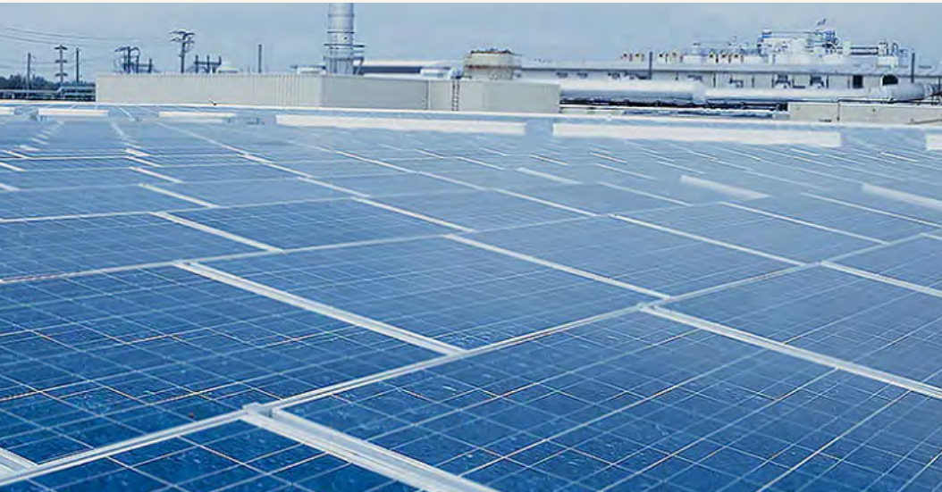
The 3.3 acres of 3,900 solar panels at our Salem, New Jersey facility generated 677,406 kilowatt hours to help power the site in 2023.
