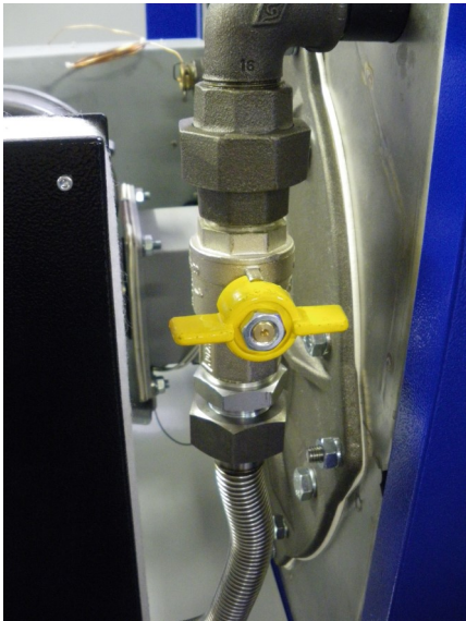
Figure 8.1.1 - Gas Isolating Valve
