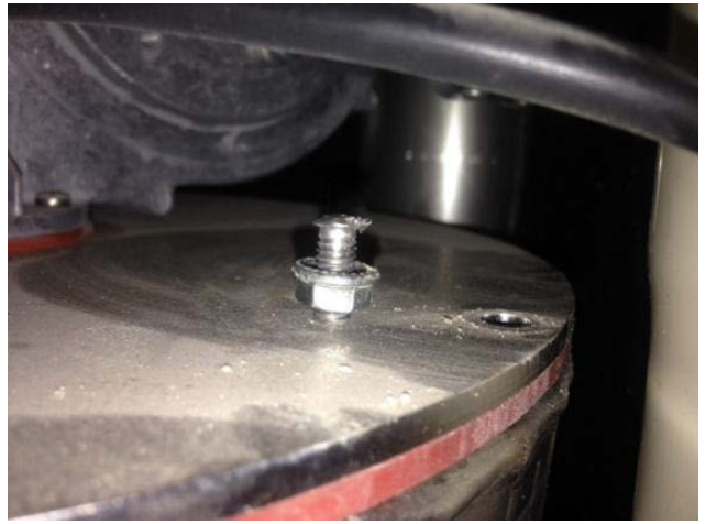
Picture showing failure mode (broken stud)
