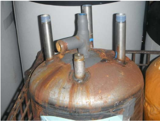
Picture showing failure mode (pin hole leak in the Excellence tank nipple connection)
