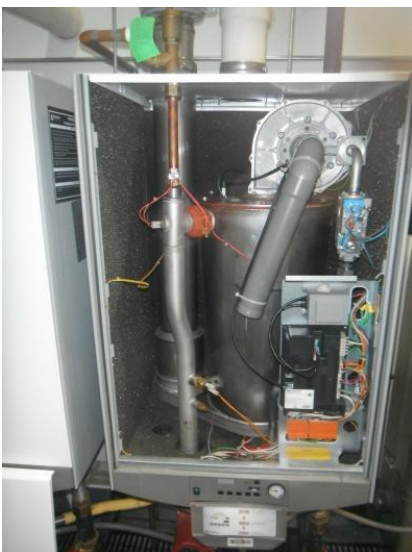
Overall photo of the boiler with the front jacket removed
