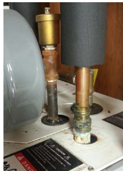
Picture showing boiler connections
