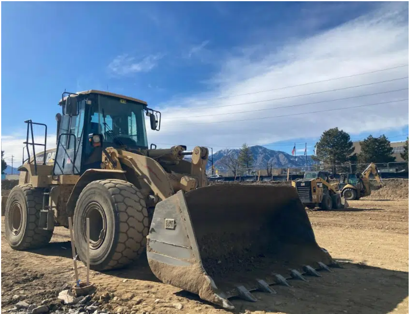
Construction equipment at a redevelopment site on Central Avenue in Flatiron Park. Lucas High/BizWest.
