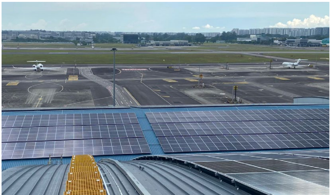
Jet Aviation's Singapore facility installed 12,000 square meters of solar panels. The panels produce energy that is fed into the local power grid and used by the site during daylight hours.
