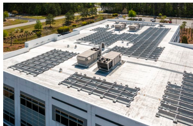
Solar installation at Gulfstream facility
