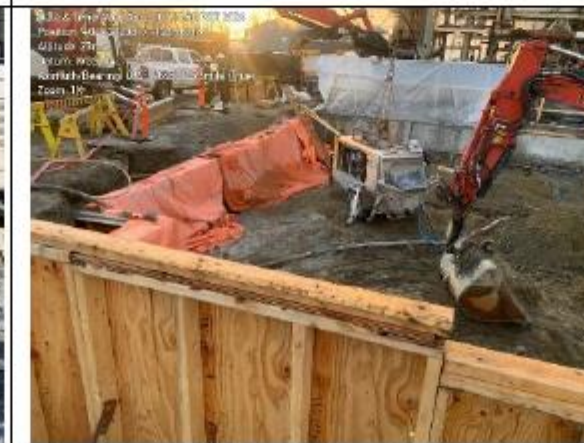
Accumulations of water must be removed
