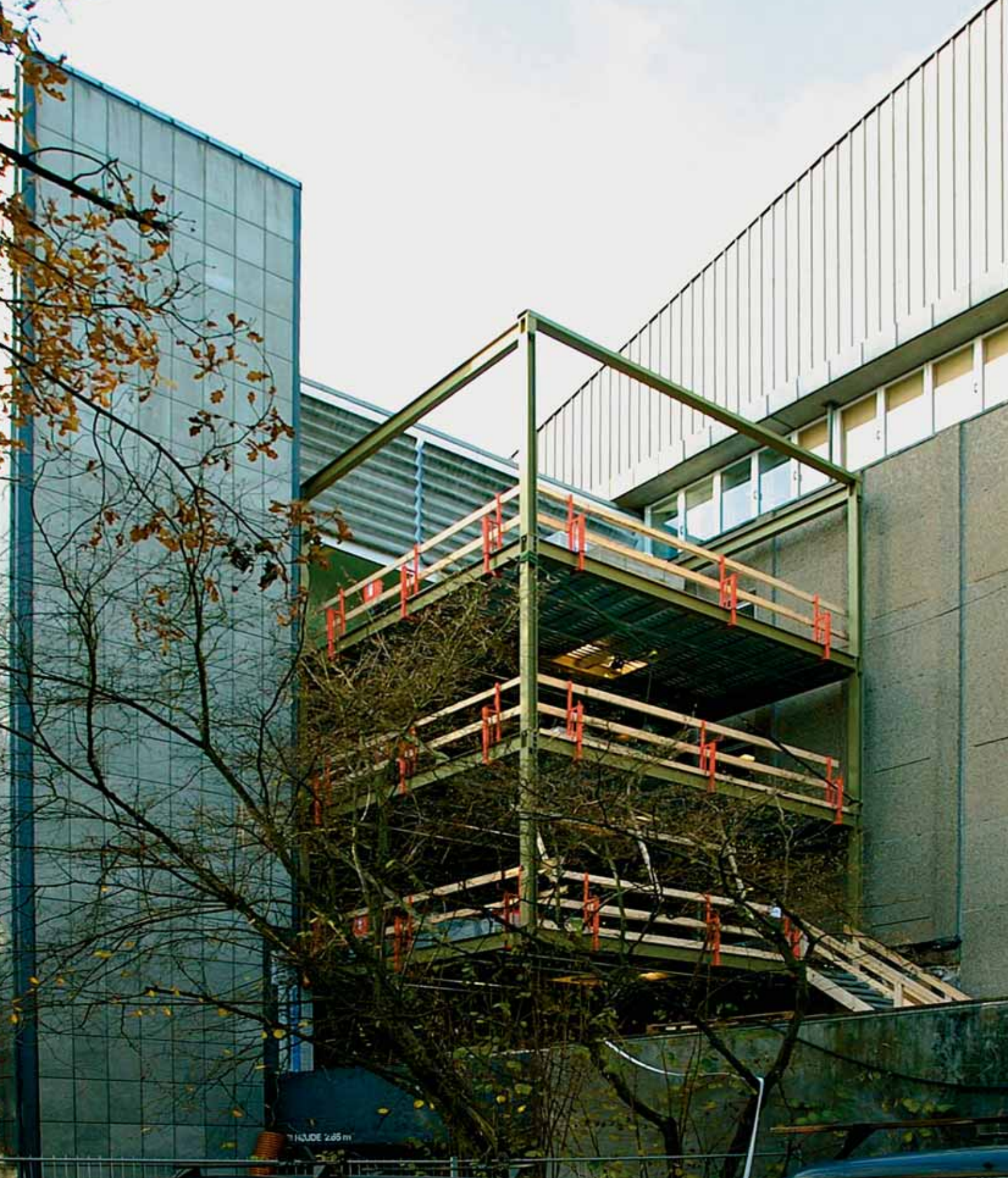
Construction on the building that will house the GBIF Secretariat was begun in September, 2002.
