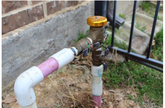
Example of above ground backflow prevention assembly.
