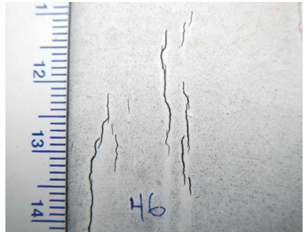
Circumferentially oriented crack field
