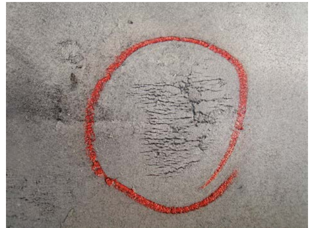
Axially oriented crack colony
