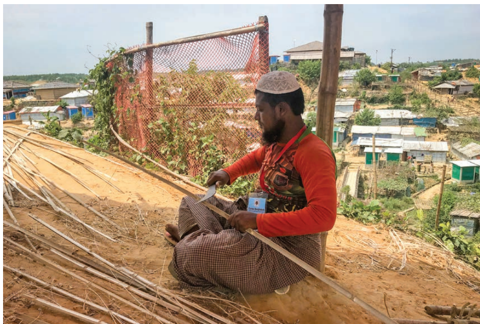
Mohammed Tayeb working at a distribution point being constructed by refugees through cash for work funded by CAFOD's DEC programme.
