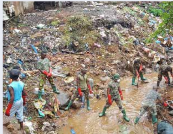
Kissy Brook bridge before the FCC clean-up
