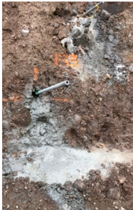
DYWI® Drill Hollow Bar installed with simultaneous drill & grout HoTV A465 South Wales
