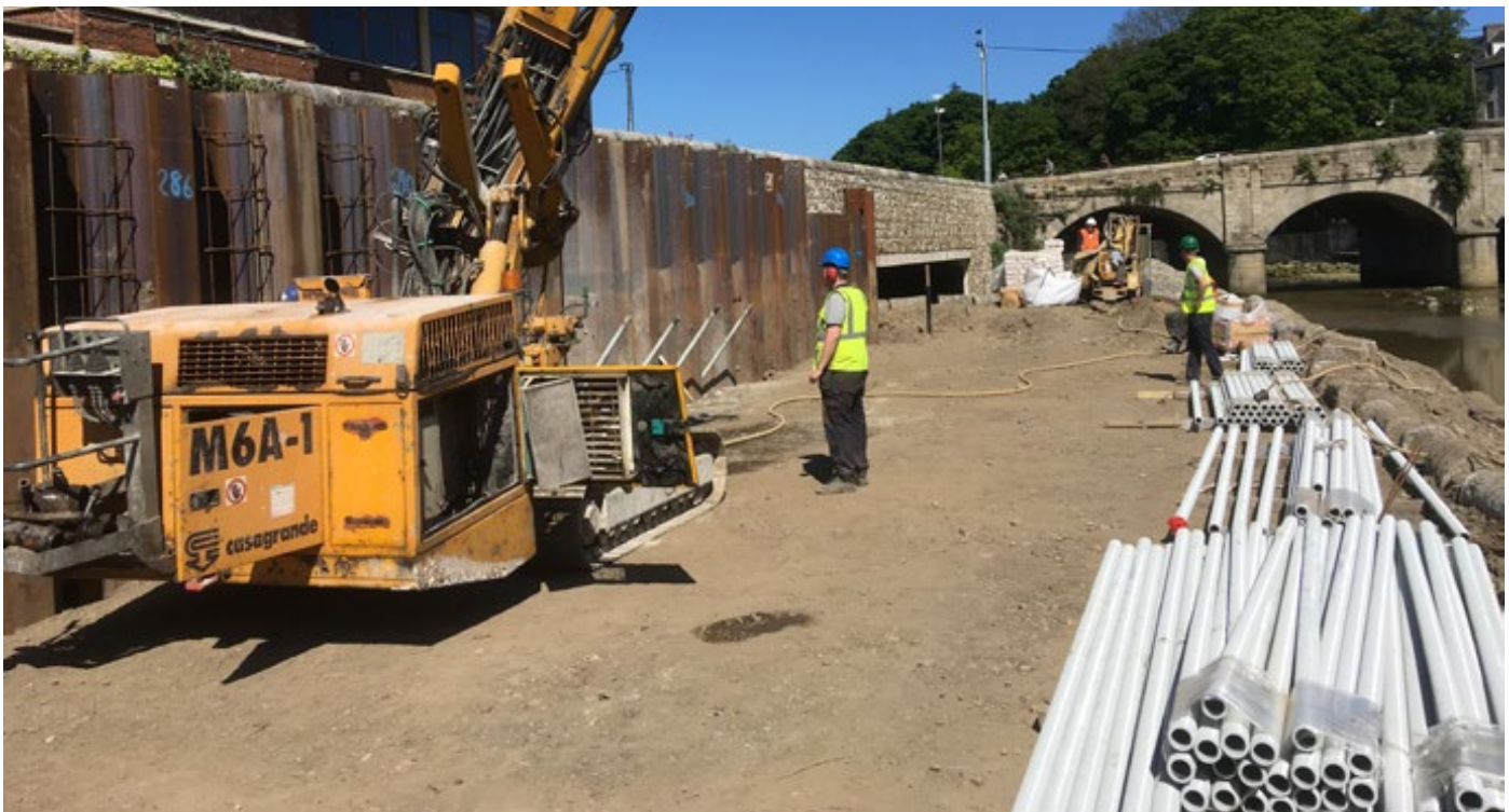
DYWI® Drill R51 Duplex coated Hollow Bar is installed on the River Dargal Flood Aleviation Scheme, Ireland
