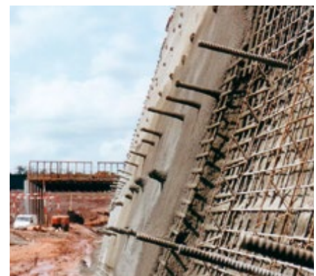
DYWI® Drill Hollow Bar shotcrete used to create a ridged face to a stabilised slope.
