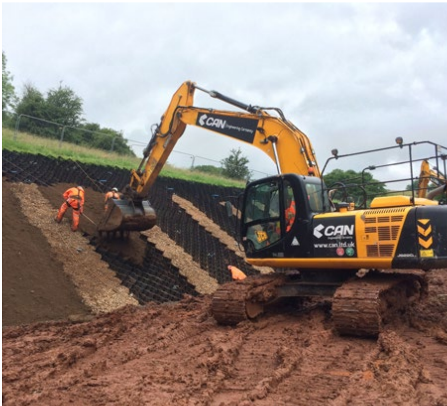
DYWI® Drill Hollow Bar & TECCO® overlaid with Geocell to retain topsoil on the face
