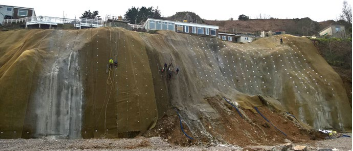
Spoil at toe left in place as erosion control and slope buttressing, DYWI® Mat Green used to prevent erosion.
