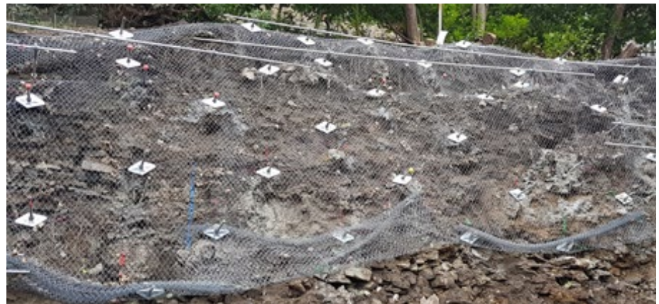
DYWI® Drill Hollow Bar & TECCO® G45/2 stabilising a new cut in Halifax
