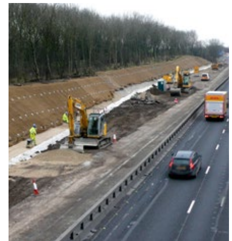
GREENAX® – Installation adjacent to the M1 Motorway, Wakefield
