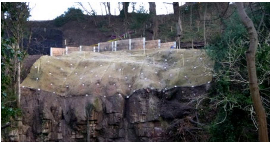
GREENAX® – Installation in Edinburgh to stabilise the loose soil overburden at the crest of a rock face
