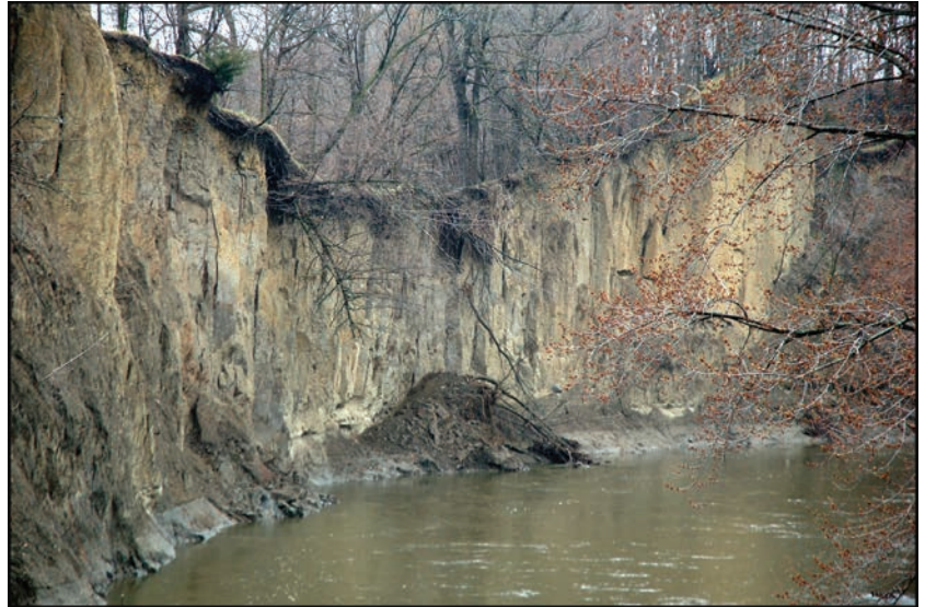
Erosion along the LeSueur River east of Mankato; photo by Carrie Jennings
