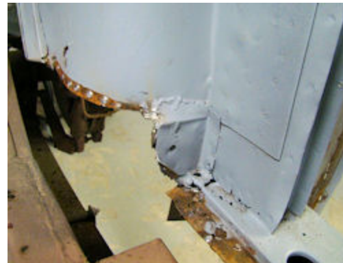
More corrosion to be dealt with
