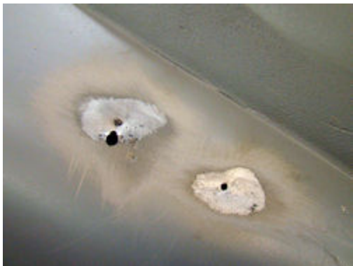
More issues hidden beneath lead
