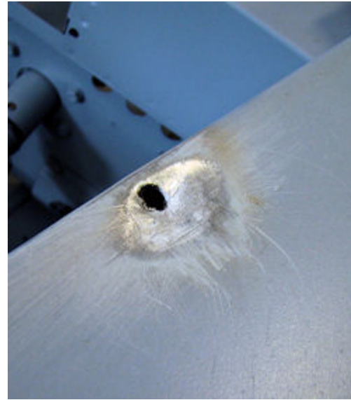
Unfortunately, lead has been used to hide corrosion at a number of locations around the body
