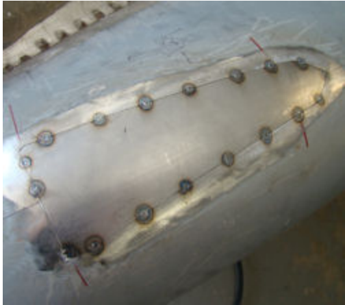
Trimmed and fitting perfectly, the new panel is first tacked into place
