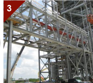
3 Cable trays take cable from the substation to process unit.
