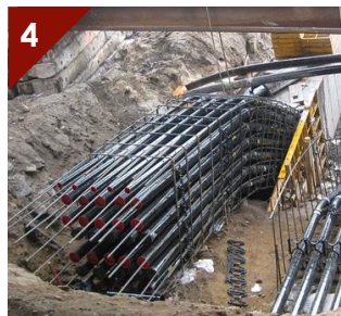
4 Conduit duct banks connect to process unit.
