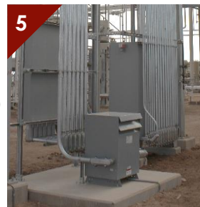
5 Conduit and cable connect to control stations, lighting, electric motors, etc.
