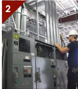
2 Substation connected to electrical control systems.
