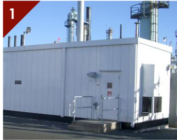
1 Unit substation act as as an electrical control center in an industrial facility.
