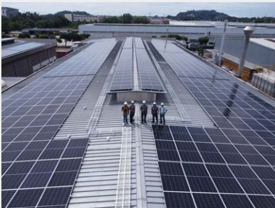
Solar panels on the rooftop of dormakaba's manufacturing facility in Melaka, Malaysia
