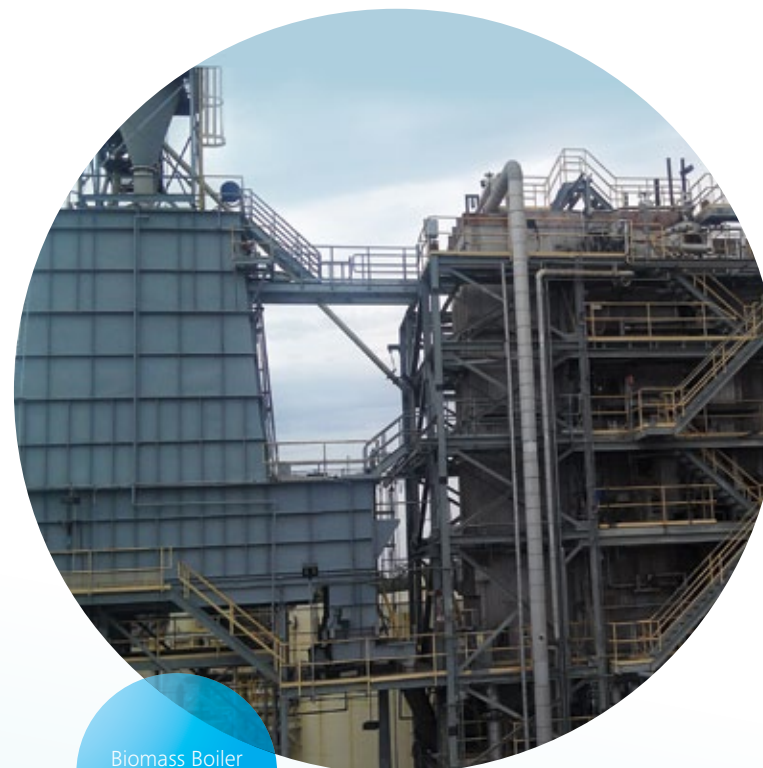
Biomass Boiler Albany, Georgia
