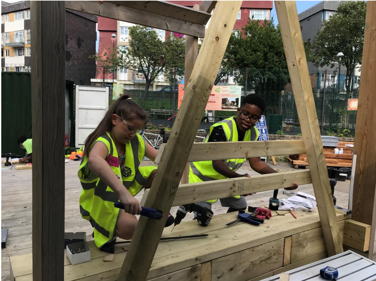
Photo: Two participants building a wooden structure with tools in Build Up London project
