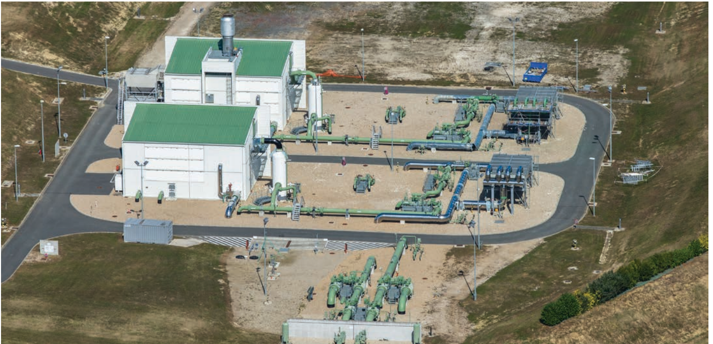
Sauveterre compressor plant
